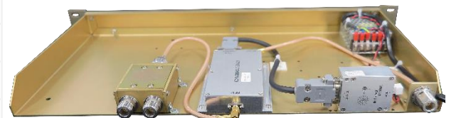
Control Unit and LNA mounted on 19-inch rack together with power supply unit and 1:2 power divider
